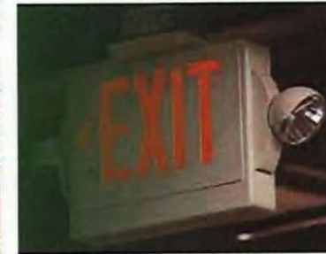
EMERGENCY & EXIT LIGHTS
