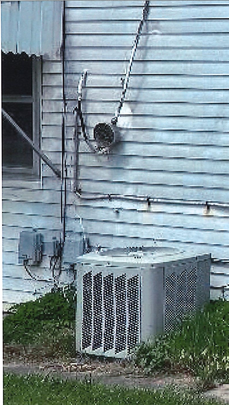
Exhibit D1.7 – Bravo Side (Disconnected Electric Meter)
