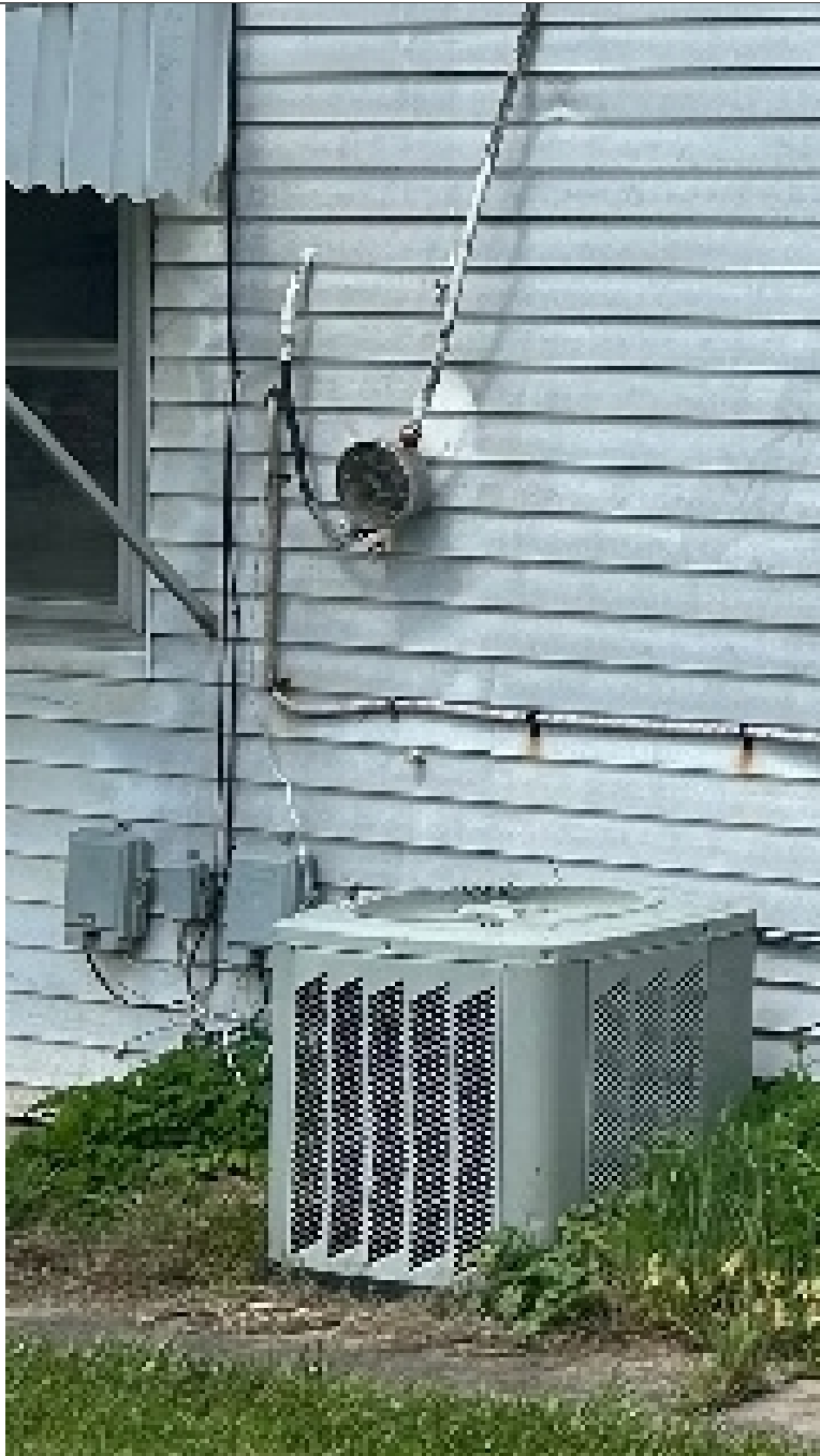
Exhibit D1.7 – Bravo Side (Disconnected Electric Meter)
